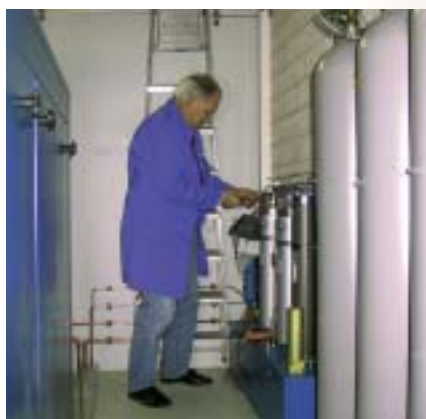
Compressor room of a helium recovery unit
